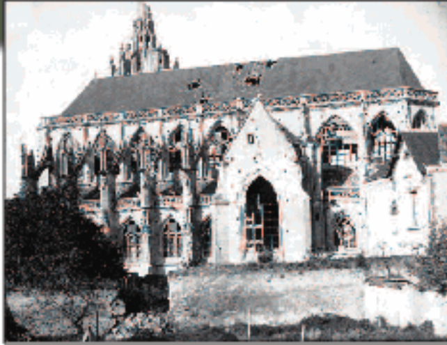
Above: Unpublished photograph of the southeastern façade of Saint-Martin Church. Although less damaged than Saint-Germain, this building's roof was pierced in multiple places and its stained-glass windows blown out by Allied cannons. (Author's collection.)
